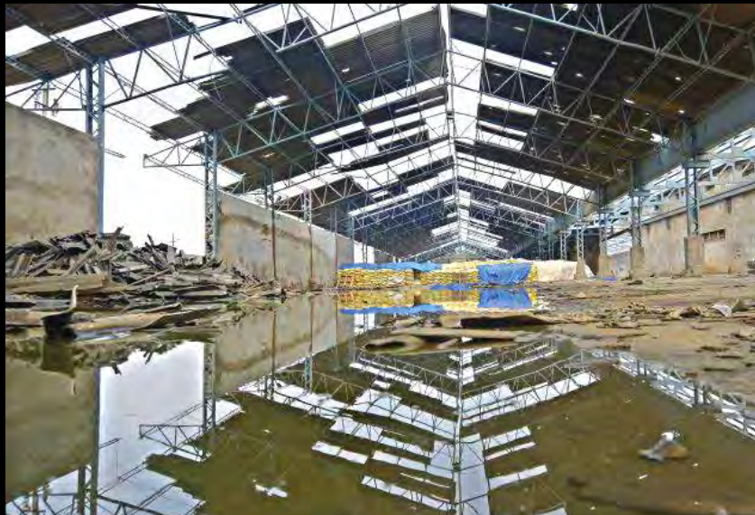
One of the severely damaged warehouses meant for storage of cargo after loading and unloading operation at Visakhapatnam Port, in the aftermath of cyclone Hud Hud
