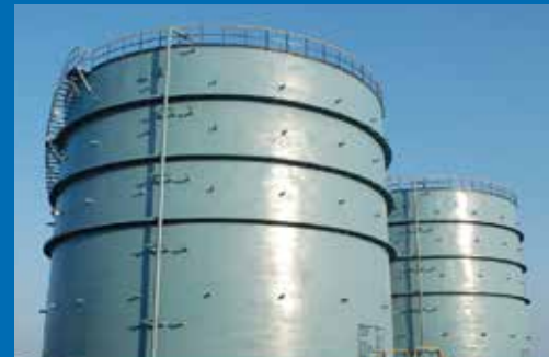
Tank farms for liquid cargo
