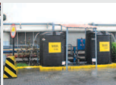
The layout of the tanks and the pumping system.
